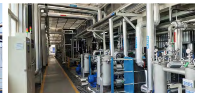
Application of air source heat pump technology
