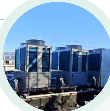
▲ Application of air source heat pump technology
